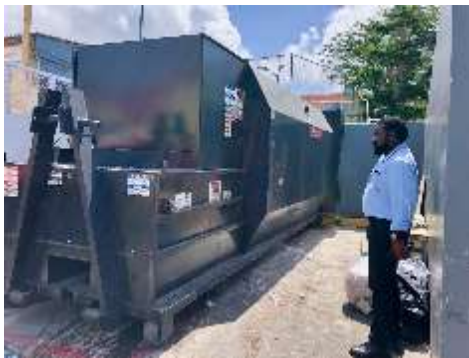
A Waste Compactor in a Resort Hotel
